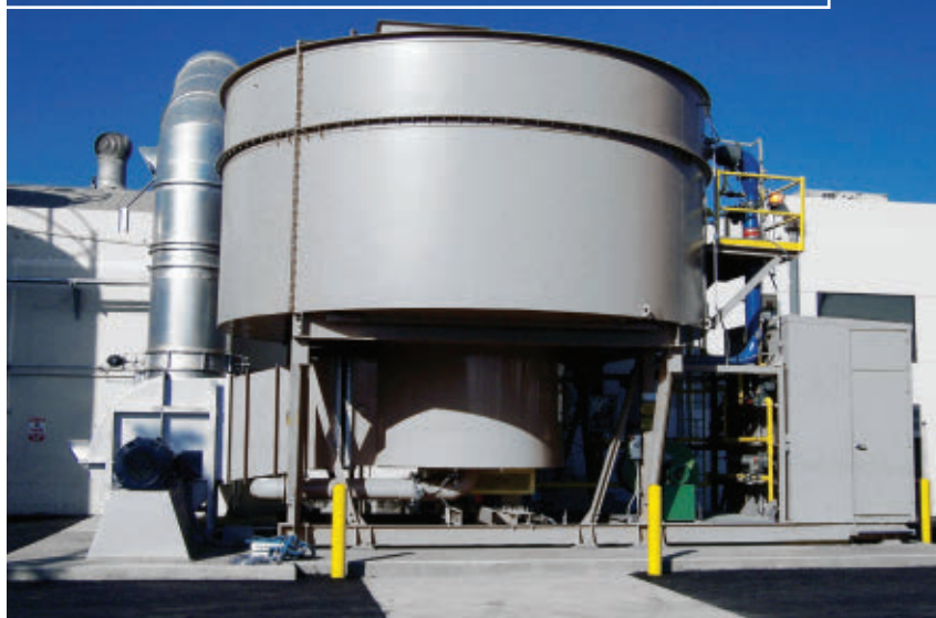
Engineered Abatement Systems for Environmental Compliance
